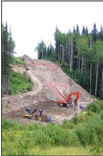
Figure 3a Landslide movement parallel to pipeline
